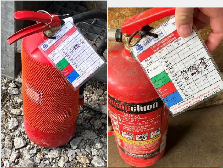
Regular inspections of firefighting equipment
